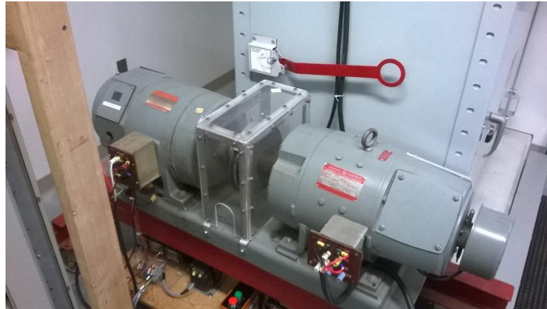
5 HP Utility Generator 3 phase 208V
