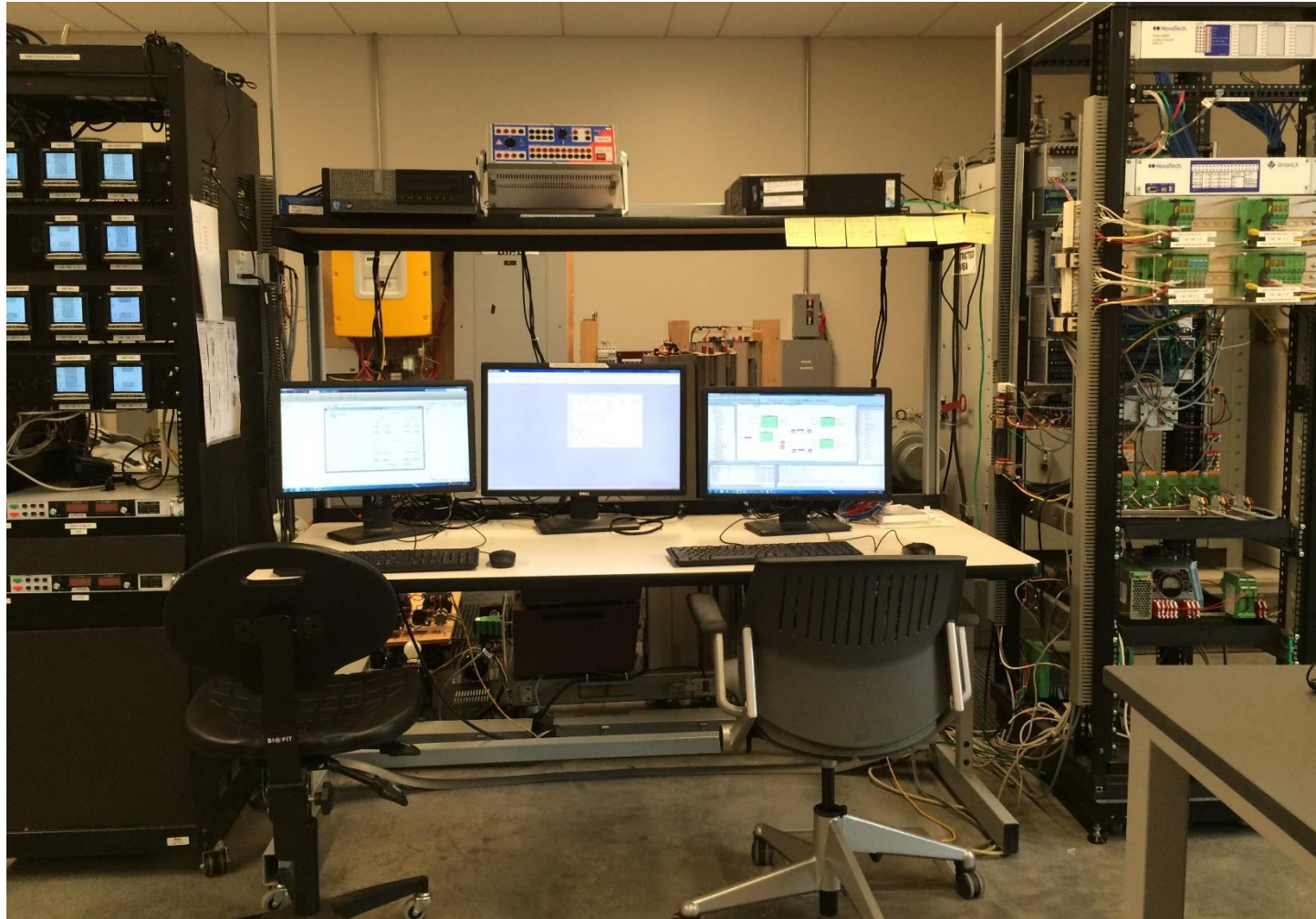
Distributed Control System Hardware
