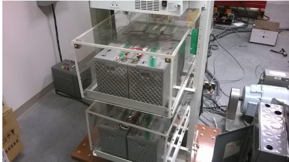
48V 180Ah Battery Bank
