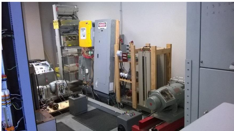
Figure 3. Right View of Microgrid Test Bed
