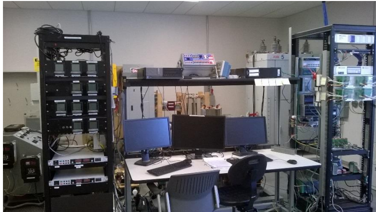
Figure 2. Microgrid Control Center
