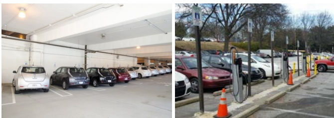
Fig. 7. Indoor and Outdoor Chargers
