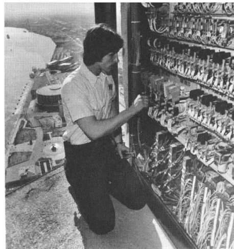
A modern controller high atop Detroit's Plaza Hotel. [Strakosch98]
