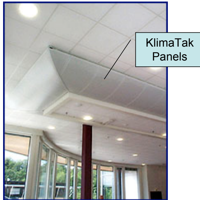
Figure 2.4: Another common KlimaTak acoustical panel. The ducts are hidden by the acoustical paneling and a drop ceiling all around.
