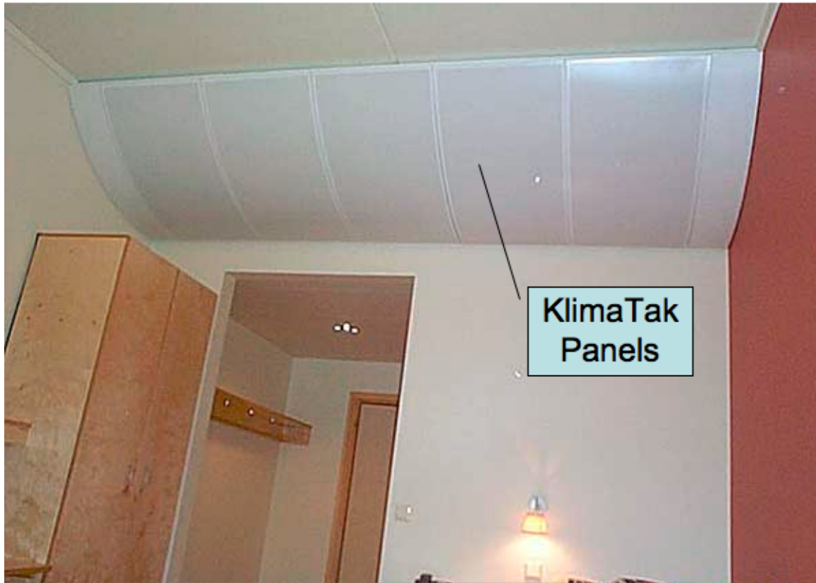
Figure 2.3: The most typical KlimaTak acoustical panels shown here in a hotel room. The ventilation duct is run behind the white sheet metal panels.
