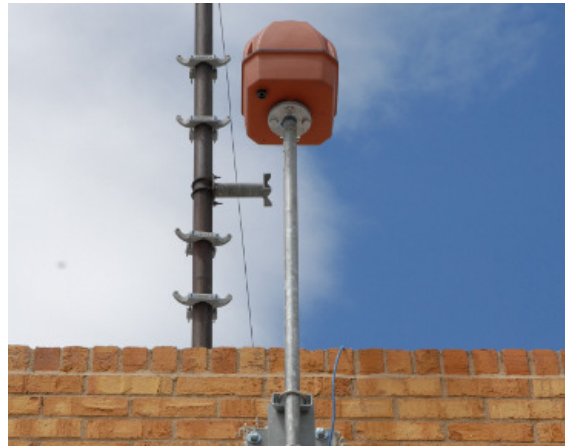
(b) Installed Antenna Node
